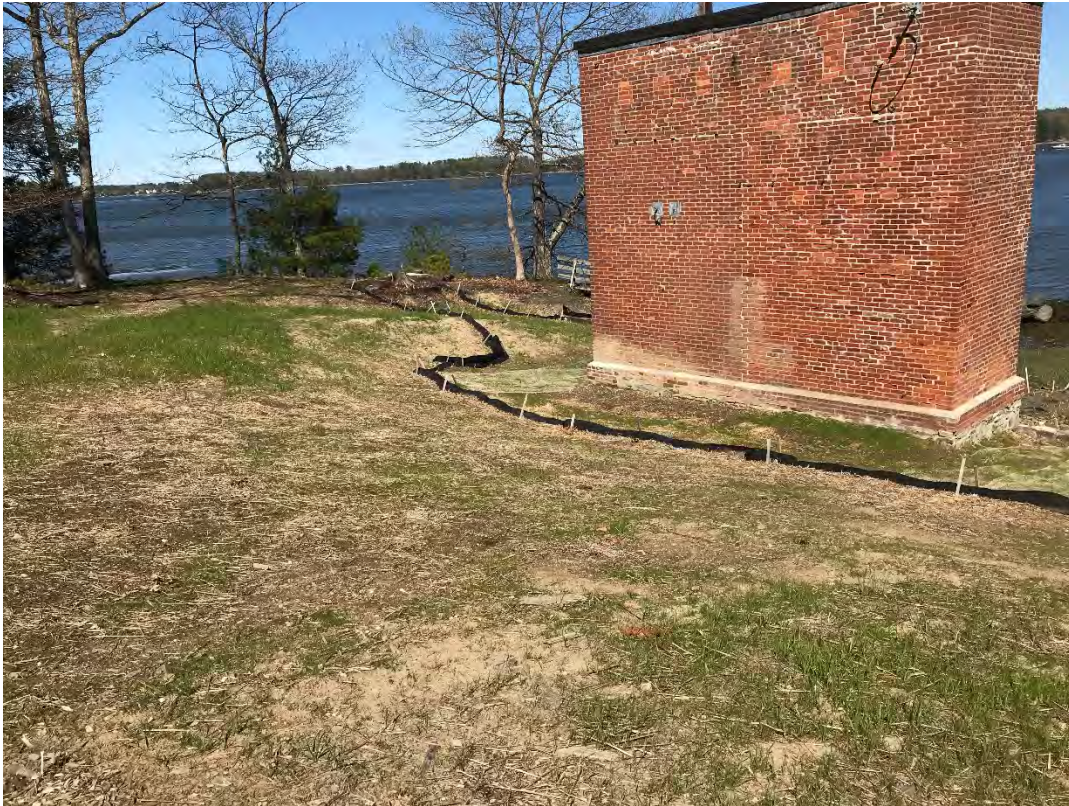
Fig 1: Slope leading down to cable house and salt marsh restoration at the west side of the bay. Viewing northeast. (05-06-21)
